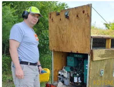
Jim, N8VIM, with his trusty generator that powered us through the weekend:
